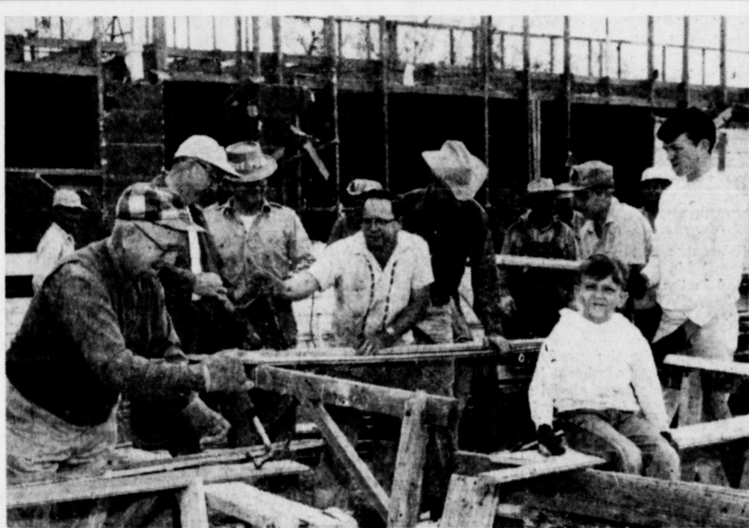
OPERATION NAIL PULL — Members of Church of Christ congregations from several areas showed up to help salvage lumber from the old Buffalo Lodge which is being torn down.
