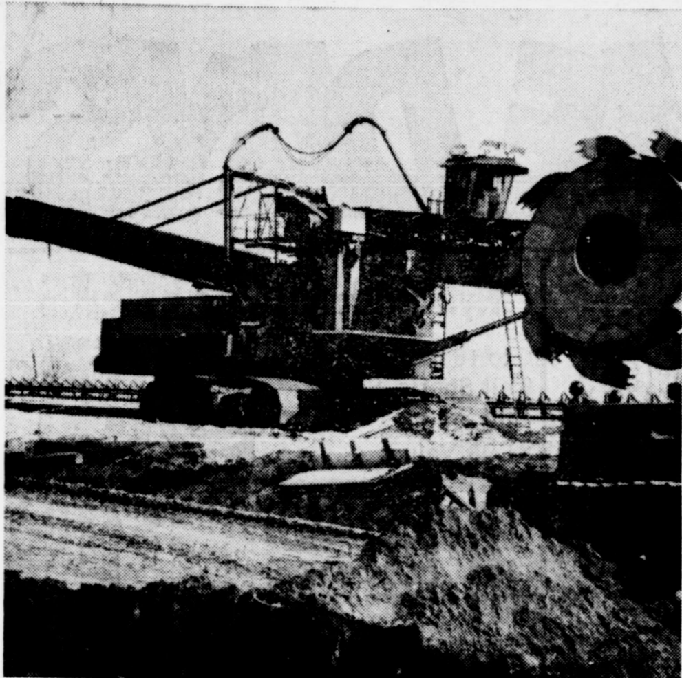
LOADED WITH POWER —Dominating the construction site at a new coal loading facility in Kellogg, Ill., is this giant called an electronic-controller-stacker. The big machine can move 3,000 tons of coal per hour into waiting river barges.
