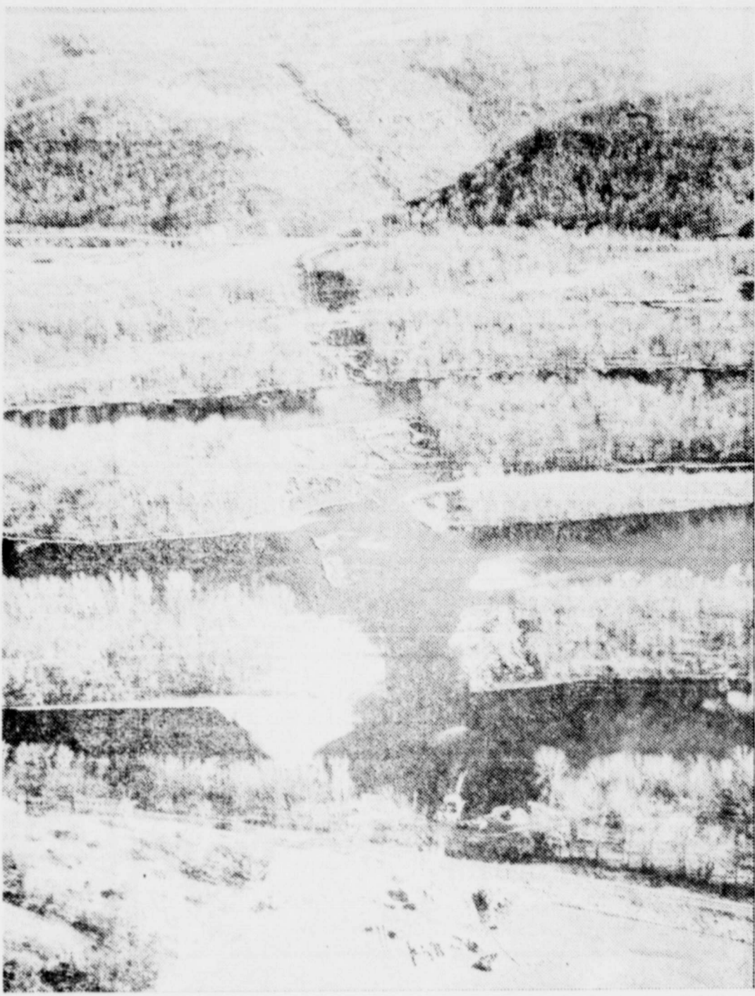
THE LONG FINGER OF MAN—Cutting a jagged swath across field, river and hillside, this man-created right-of-way for a gas pipeline in Washington changes nature but will provide for human needs.
