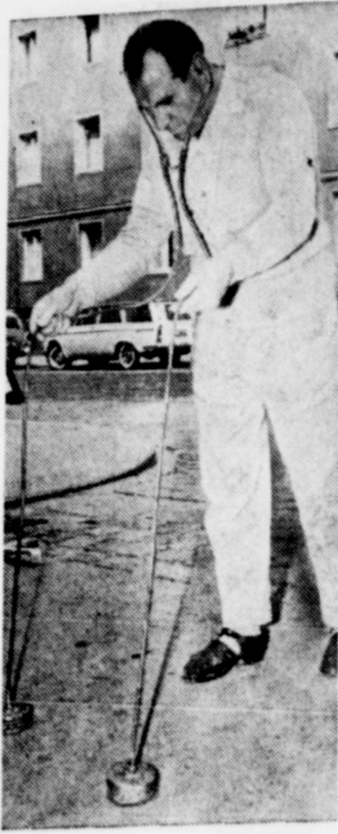
EAR TO THE GROUND— Listening with his "geophon," this expert from the Vienna, Austria, water works searches under the street for defects in the piping, 30-feet below.
