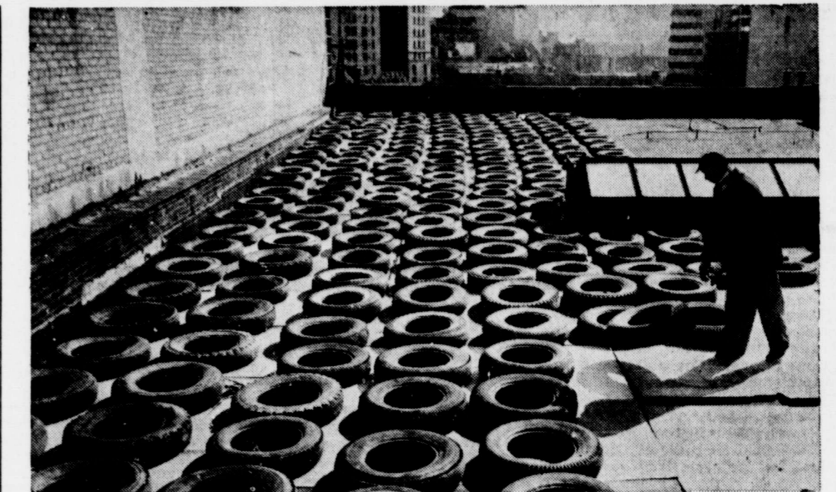
TIRING WORK —Worker lays down hundreds of rubber tires on a Rochester, N.Y., rooftop. The old tires and plywood sheeting are used as protection against falling debris from the adjacent building being torn down.
