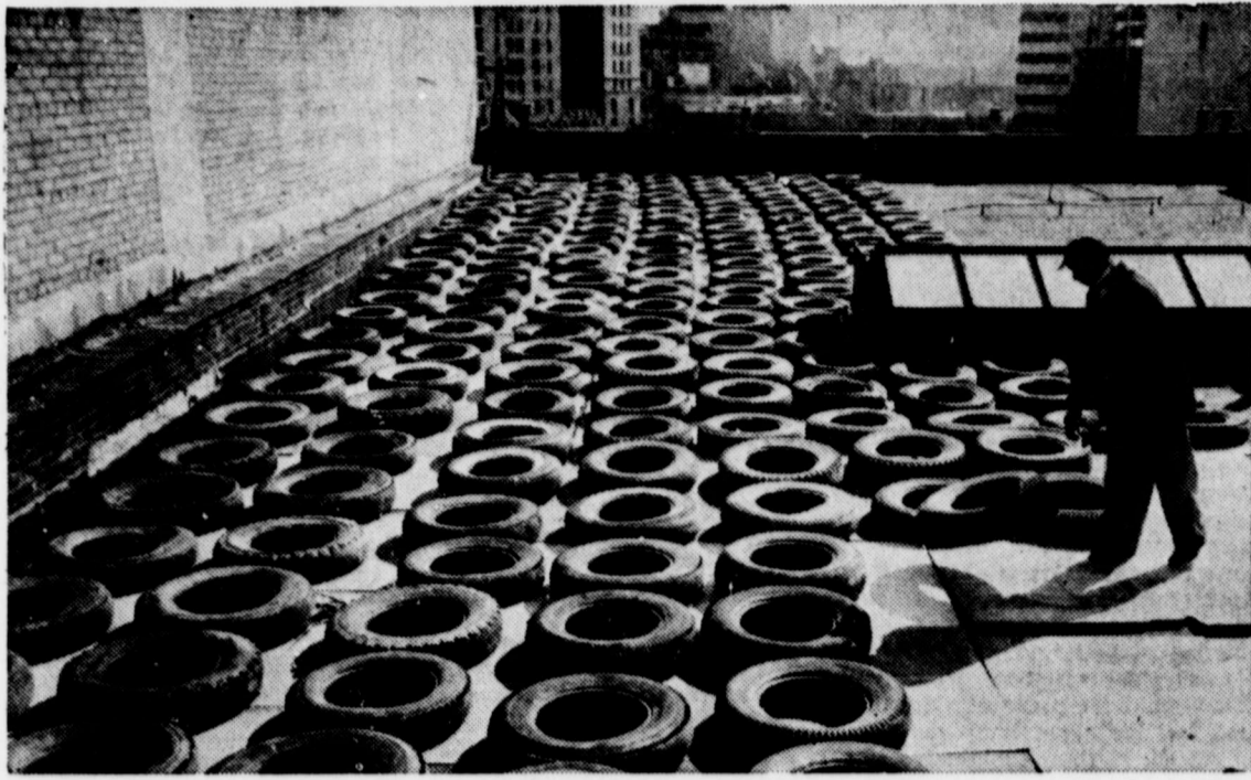
TIRING WORK—Worker lays down hundreds of rubber tires on a Rochester, N.Y., rooftop. The old tires and plywood sheeting are used as protection against falling debris from the adjacent building being torn down.
