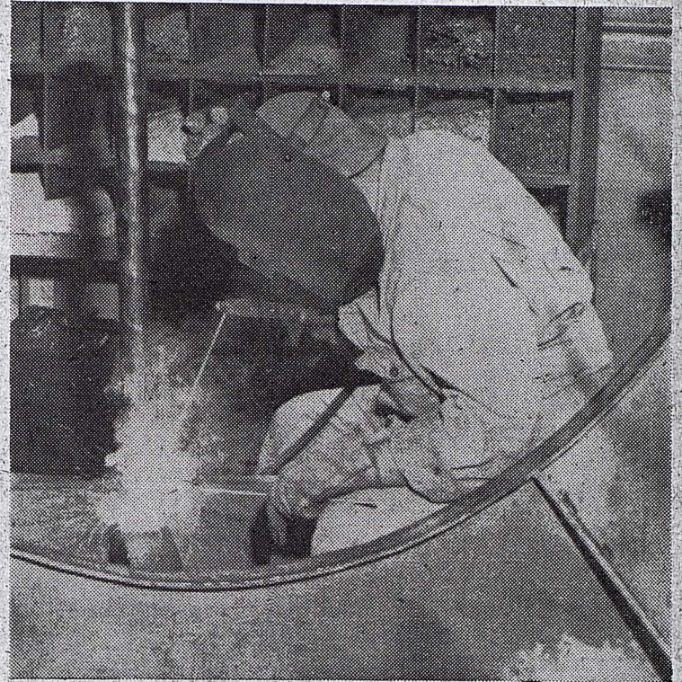
ONE OF THE BEST . . . That's what Navy inspectors said about "Rocky" Barilla, Brooklyn welder, a couple of years ago when he passed his examination as a certified pipe welder. Now Pvt. Rocco Barilla is carrying on in his welding trade for the Army. Some of the work he does now is simple compared to the tough jobs that must go into the construction of ships.
