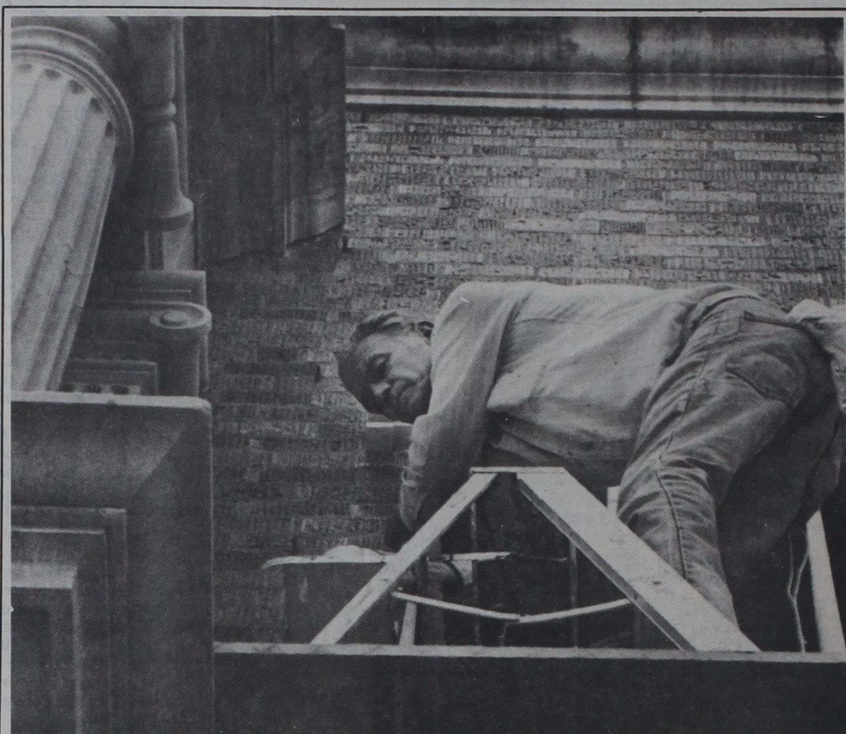
'Stoop' Ladder Maintenance man Dennis Duncan puts added touches bars on the second story windows of the Science Building. Here, Duncan is painting the
