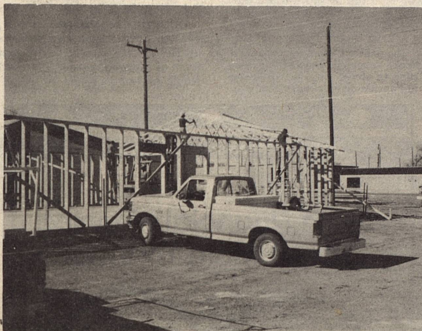
BAYER LUMBER REBUILDS -- Milton Bayer, owner and operator of Bayer Lumber states "he hopes to be operating out of the new facility by mid-April." The original building was completely destroyed by fire in December, 1987.
