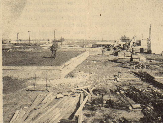
The vocational training building being erected by the Plains Independent Schools is well underway. Being done in a series of operations, the floor of the 1st section is being poured to-day. Brick laying will follow next week.
