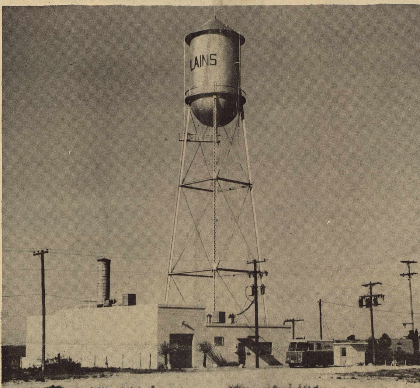
Du Pont Desalting Water Plant. Installation here processes 100,000 gallons of good quality water per day through "Permassep" permeators and places it in the municipal distribution system.
