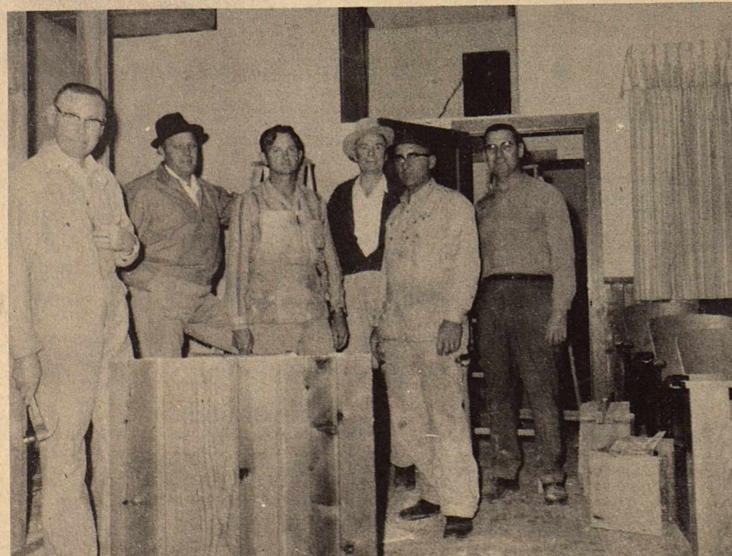
REMODELING: Men of The First Baptist Church recently started work of remodeling and redecorating the auditorium of the Church. Plans includes wall panels, new ceiling and lights. Also to remodel the choir loft, pulpit, new windows and carpeting. The church hopes to have most of
