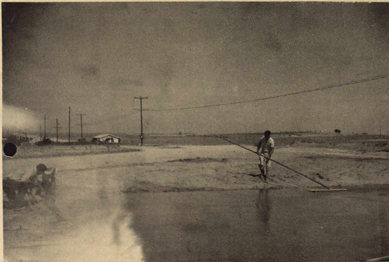
SCOUT HUT CONSTRUCTION---is now underway in complete earnestness, as the forms have been erected, the plumbing roughed in and the concrete poured. Above
