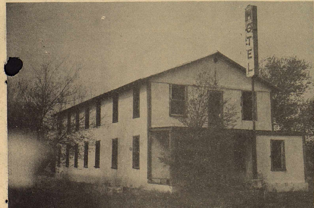
CONDEMNED--The old hotel located just one block off the square here, which has been described by many as being a terrible eyesore, is soon to be torn down according to local officials who state condemnation suit has been begun.
