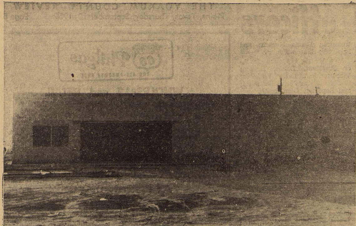
RAPIDLY NEARING COMPLETION is this modern building which will house a new grocery store. J. S. Wagley, a Plains businessman for several years, is constructing the building and hopes to have his modern grocery store open within 30 days. REVIEW Photo
