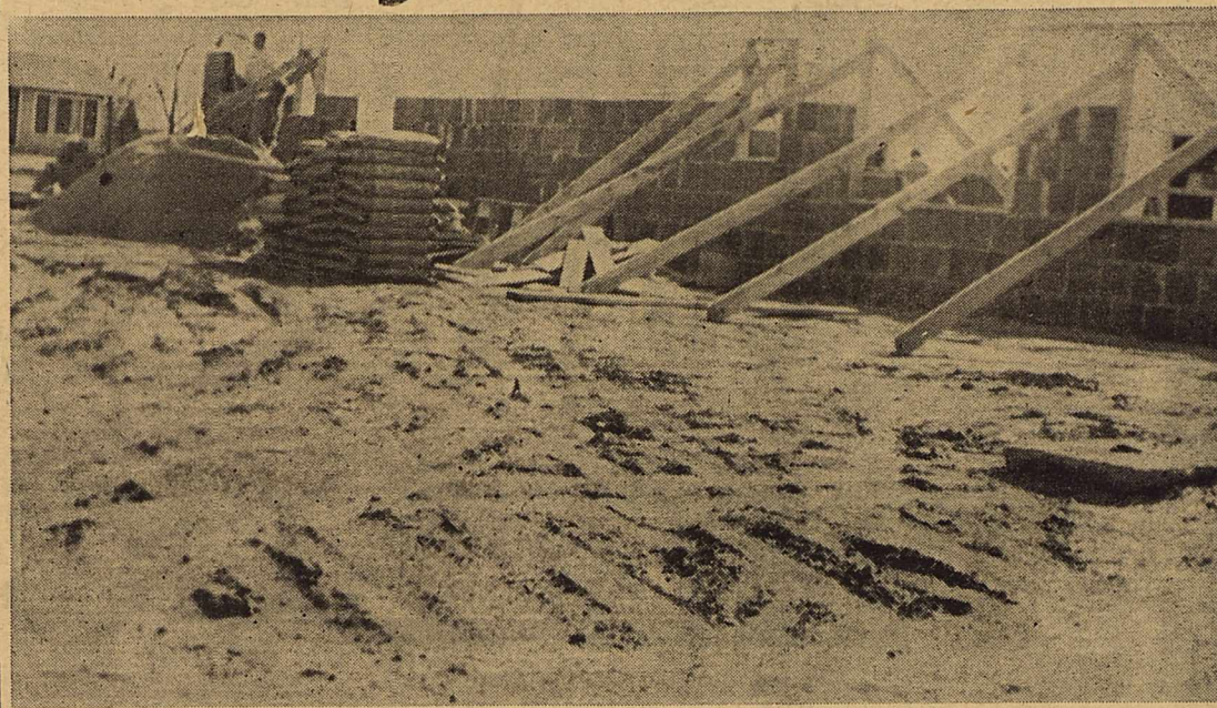
WORKERS ARE BUSY laying brick tile for the new cafe which will be operated by M. W.
