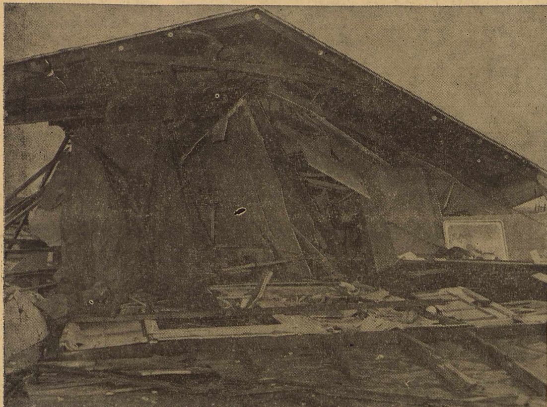
A TUMBLING MASS OF BOARDS was about all that remained of the Pressley White home following a twister which dipped down Friday night, lifted the house from its foundation, and then dropped it with a crash. —Press Photo
