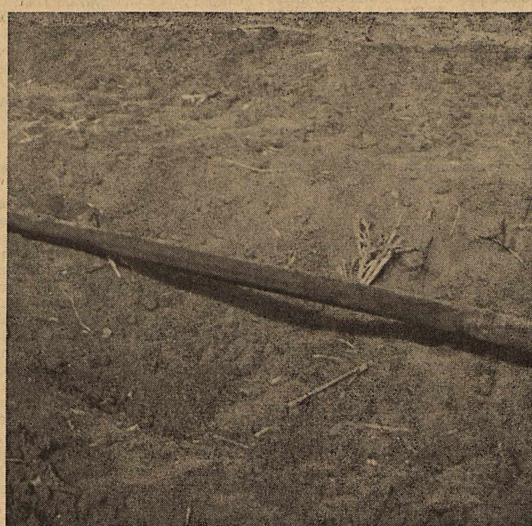
Repairs to the main gas line, broken Tuesday morning while deep plowing was being done in the field of G. R. Todd was made by putting in a new section of pipe shown above.
