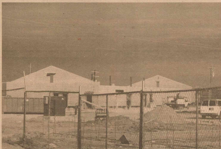
Crews continue work on the new field house located at the northeast end of the Coyote stadium.
