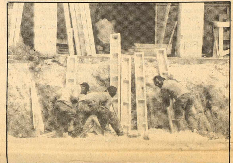
Pictured above are workers from Gary Pool Company out of San Antonio. Construction began on the Kinney County Pool last week. The City received Grant money to rebuild the pool and the construction cost is estimated at $98,000. Kinney County crew prepared the pool area for the construction company.
