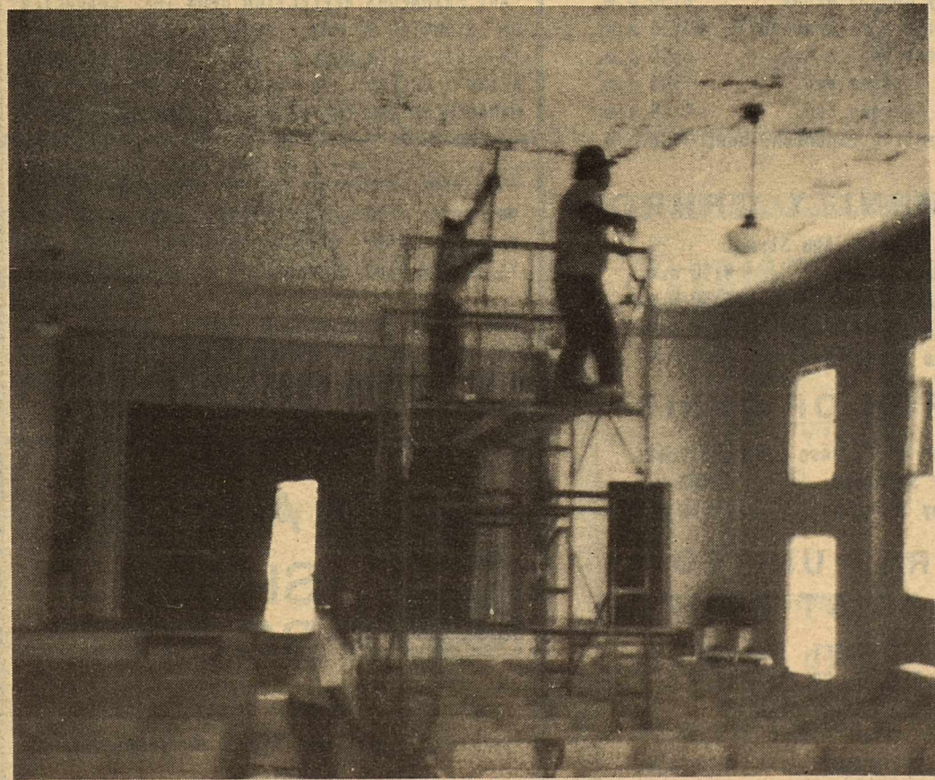
Workers for Bizzell Construction have started tearing down the old ceiling at Brackett ISD Auditorium to replace it.
