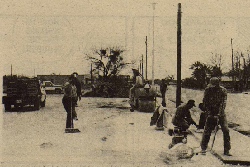
Left: Brackett Volunteer Firemen are hard at work completing the new fire hydrant which is located at the Civic Center. The firemen, along with the city, county and the highway department pulled together in the addition of this new hydrant.
