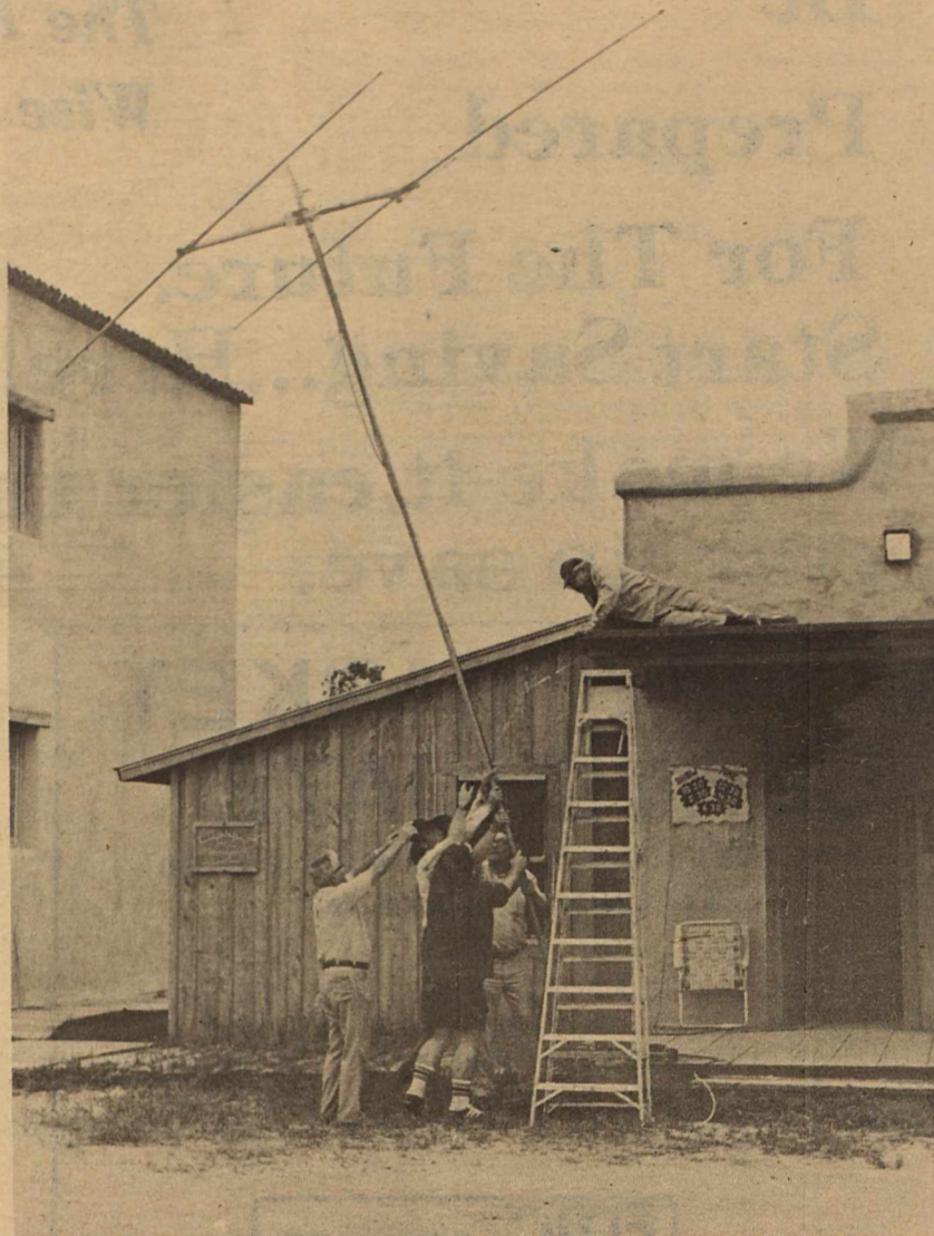
THE OLD & THE NEW....A modern communications antenna goes up in front of the Old Alamo Village Jail as the Radio Amateurs set up a simulated Emergency situation.
