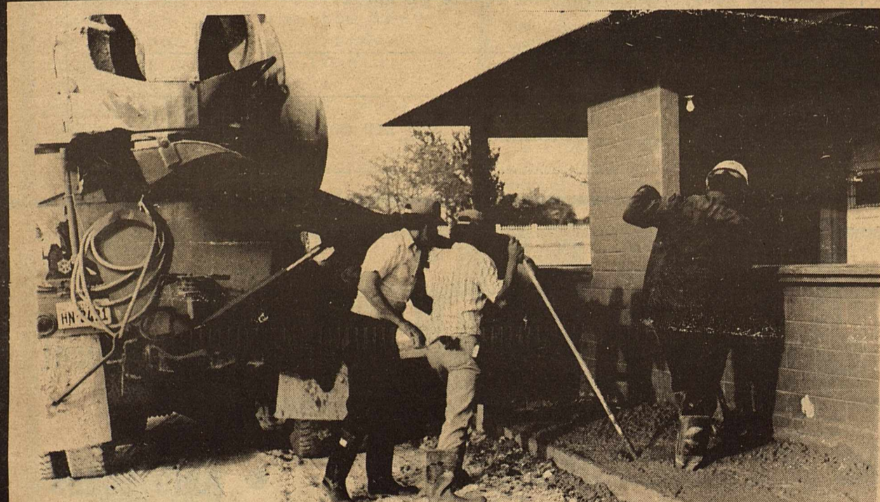
Sidewalks around the concession stand of the Little League Baseball diamond were being poured Wednesday afternoon by the Kinney County Construction Company and Baker Construction Company. This is just another step toward the improvement of our community.
