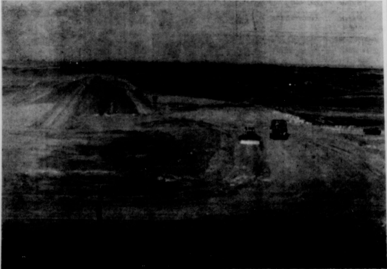
ALMOST COMPLETE—This is a picture of Site 3 dam in the Lakeview Watershed on the Lawrence Hagy Ranch northeast of Brice. This dam is 100 per cent complete on dirt work but yet remaining is the riprap with rock and fencing and adding vegetative cover.
