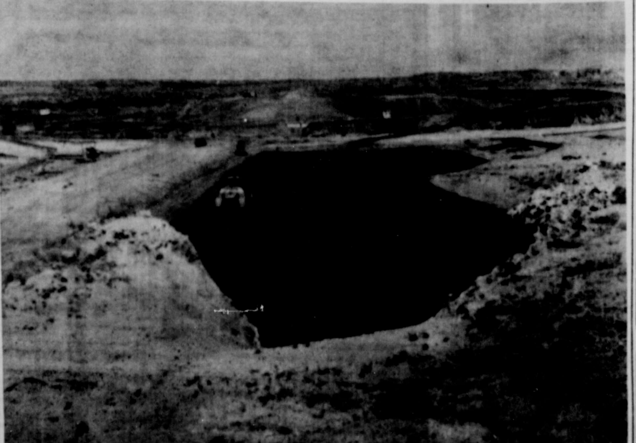
SITE 5 DAM—This picture was taken straightdown the line of the top of the 50-ft. high dam when all the dirt work has been completed. This dam will have a high storage level due to permission granted Mr. Hagy to impound more water by special request.
