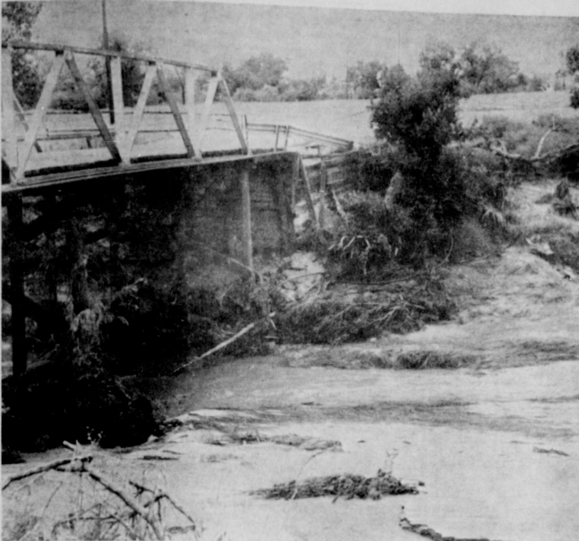
BIG QUESTION —City Officials are concerned if there has been structural damage to the City Park bridge, and considering what went by the bridge last Friday, they have good reason. Highway engineers will be here Tuesday to examine this and many other bridges in this area. County and City governments are seeking disaster relief.
