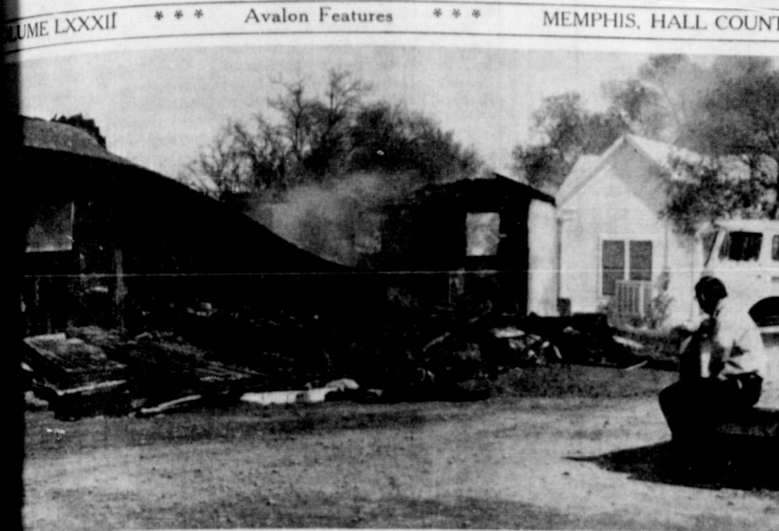
DESTROYED BUILDING —Pictured above is the J. D. Evans Store on North 16th Street as it looked Wednesday morning following a 2:15 a. m. fire which gutted the structure. The building owner is Paul Hancock of Clarendon. He reported the building was un-insured. Hancock had the building under lease and was operating a discount supply store, and using the store to park his used cars. On the right is pictured Fireman Charles Waller who is watching over the smoldering frame remains.
