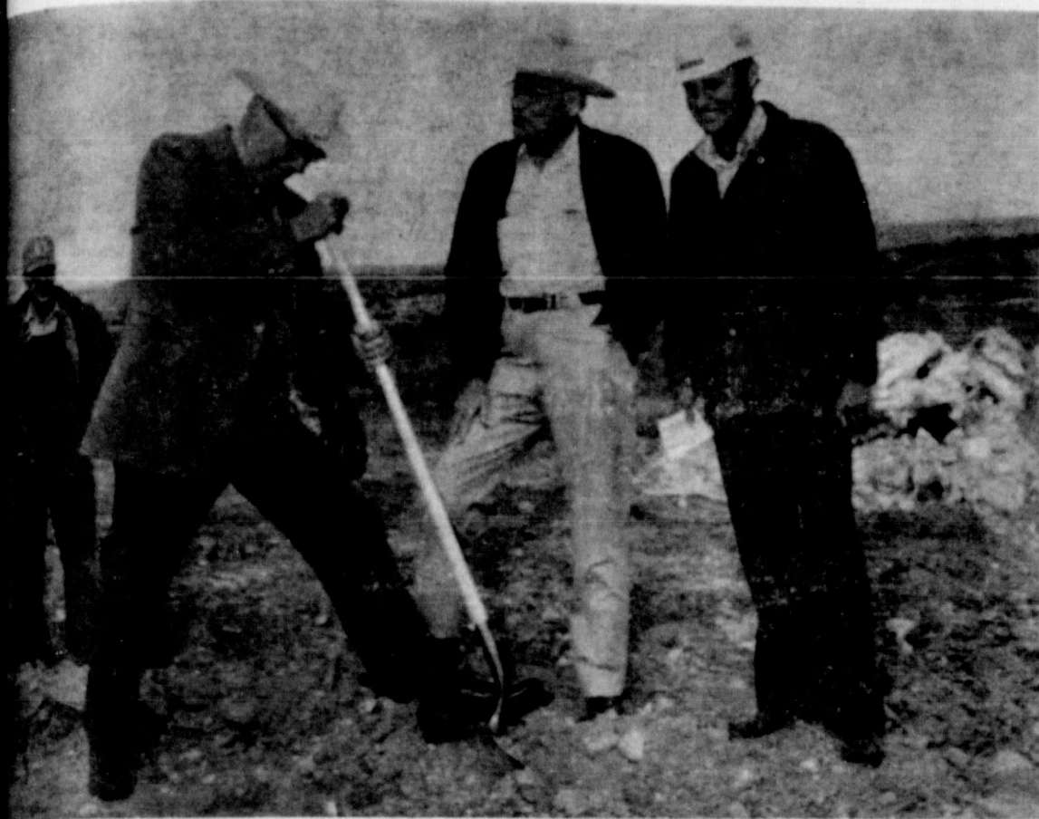
GROUND BREAKING —Pictured above, Paul Montgomery is shown turning a shovel during ground breaking ceremonies Wednesday at Site 4, Lakeview Watershed. Giving encouragement is L. R. Hagy, ranch owner. Contractor Byron DePauw (right) was host to group on a tour of the construction site.
