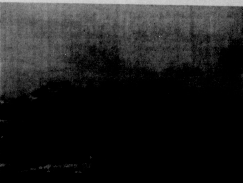
SALVAGING WASTE MATERIAL — Above is pictured crushing plant in Hartley County where an old abandoned runway is reused as base material for paving on U. S. Highway 54. This is an example of cooperation between road builders and the Texas Highway Department.
