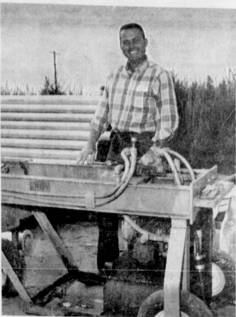
PIPE PRESS—Asst. Manager of Golden Spread, Don Davis is shown with a portable pipe press rig the firm uses.
