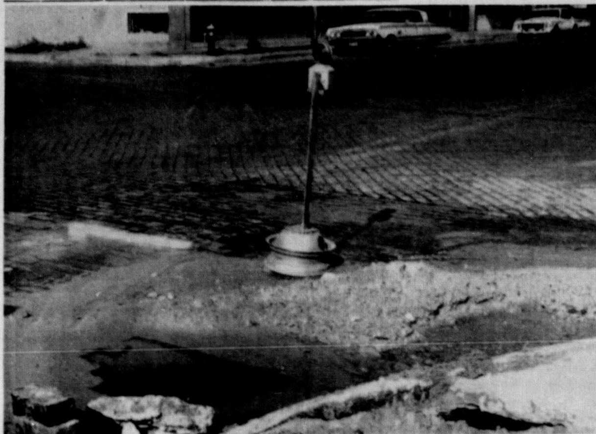
WATER MAIN TROUBLE —The crew of Donley County WCID, which supplies Memphis with water, were busy this week splicing an 8-inch water main at the corner of the U. S. Post Office which made an artesian spring when it broke through the pavement. A 6-ft. section was spliced into the cast-iron pipe by Wednesday afternoon, stopping the leak. The hair-line crack appeared to be an old one, Frank B. Foxhall reported.
