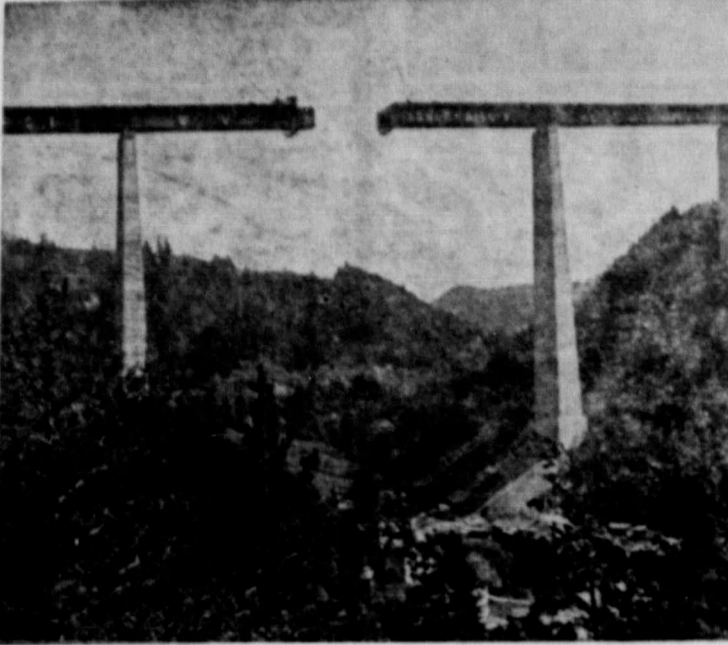
SPACE GAP . . . Inch by inch, the remaining gap of the lofty Europa Bridge spanning the Sill Valley in Austria is being closed. At this point, the opening is still almost 80 feet across. Meeting place is over 600 feet high.
