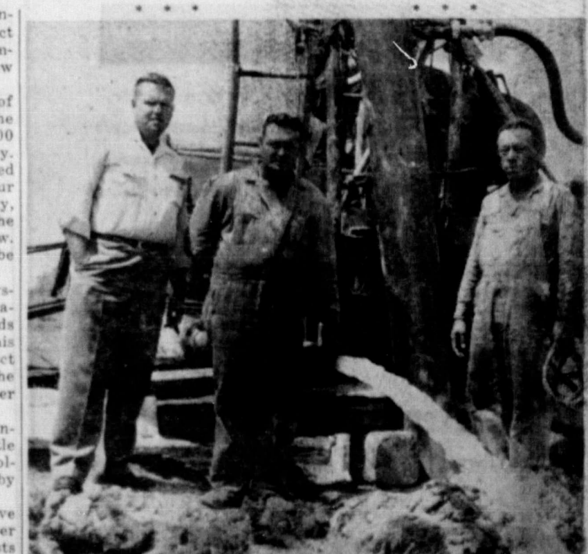
NEW WELL — Frank B. Foxhall, left, is shown inspecting the new well as it began pumping Wednesday. Others shown are R. W. Sale, center, and Lee Sisdro, both members of the drilling crew.
