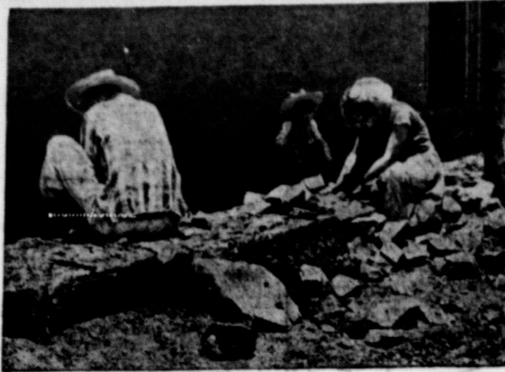
DO-IT-YOURSELF PROJECT . . . Family in Talsintuan, Mexico, constructs a sidewalk outside their home. Home improvement project is part of a rural social welfare program of the Mexican government.
