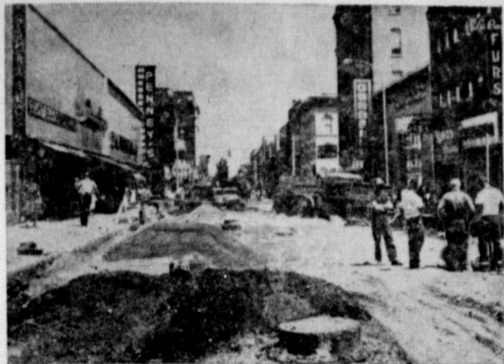
ADDING TO THE MALL . . . In Kalamazoo, Mich., workmen are busy constructing a block-long addition to the city's downtown mall at a cost of $24,000.
