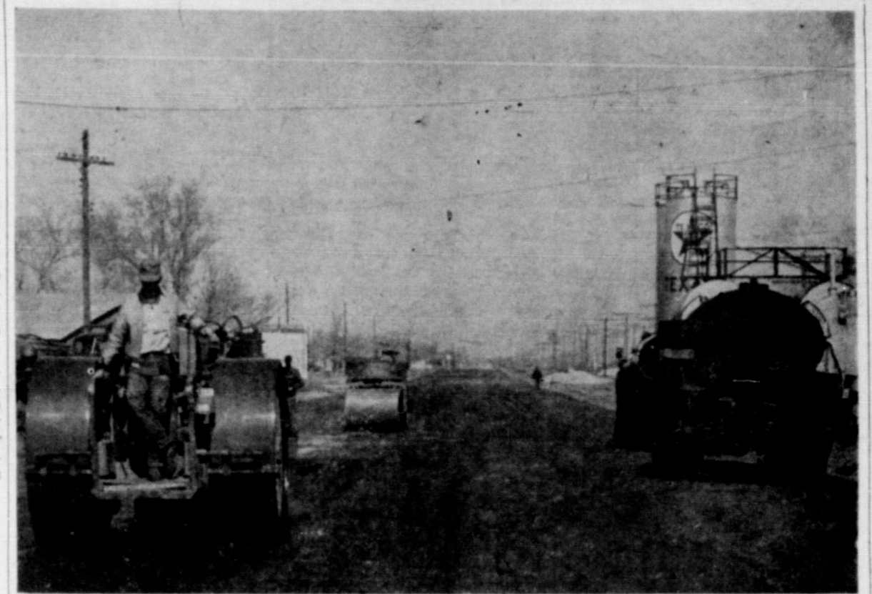
WORK ALMOST COMPLETED — Packers are shown above finishing the paving of Boykin Drive, formerly Front Street, as the construction crew lays the last strip of paving on the street itself Tuesday. Bad weather called a halt to the work Wednesday but the road will probably be ready for use about the first of next week.
