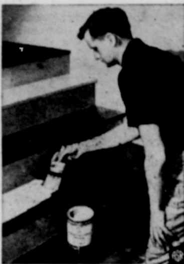
PAINT ALTERNATE STEPS to keep stairways usable while they are being painted. Finish the job when the steps painted first are dry.
