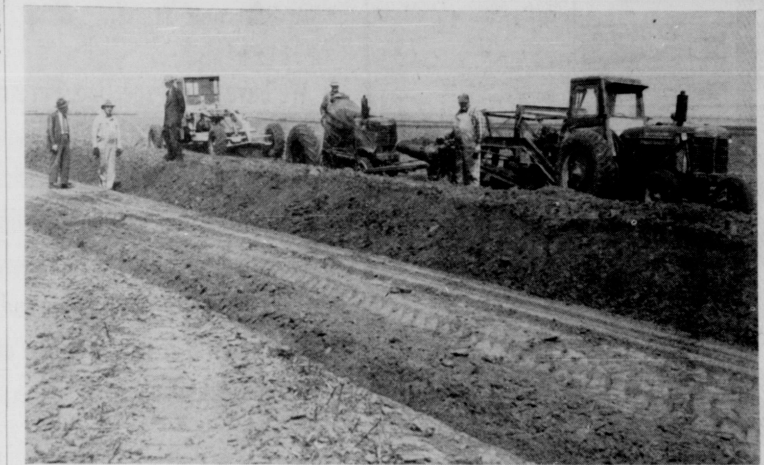
OVER THREE MILES OF NEW TERRACES A DAY are being built this week by Nat Bradley, contractor, on the Old Blades farm, southwest of Eli, which was bought this winter by Dr. R. E. Clark. The first machine in the above photo is the big elevating grader which is being operated by Barney Floyd, who has helped Mr. Bradley for several years. The second machine is a whirlwind disc tractor with L. G. Rasco sitting on the driver's seat. The third machine is a maintainer grader which is used to finish the terrace. Secretary Lynn McKown of the ACA office is at far left, talking to Mr. Bradley, while Nugent E. Brown, news editor of The Democrat, is standing atop the terrace. Photo by Wise
