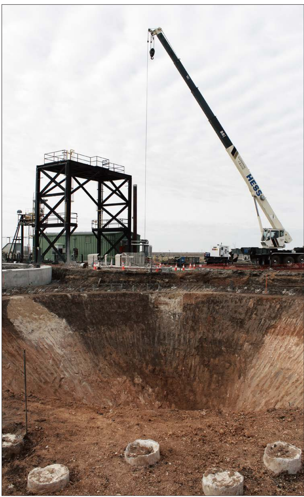
Photos by Lindsey Tomaschik Rampa, Inc. is the new tenant out at Pampa Energy Center. Construction began in early to mid-December on two new grain elevators that are expected to be completed and operating in June.
