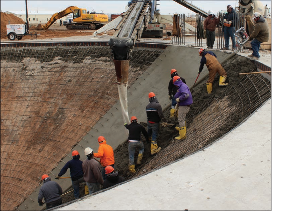
Photos by Lindsey Tomaschik Rampa, Inc. is the new tenant out at Pampa Energy Center. Construction began in early to mid-December on two new grain elevators that are expected to be completed and operating in June.
