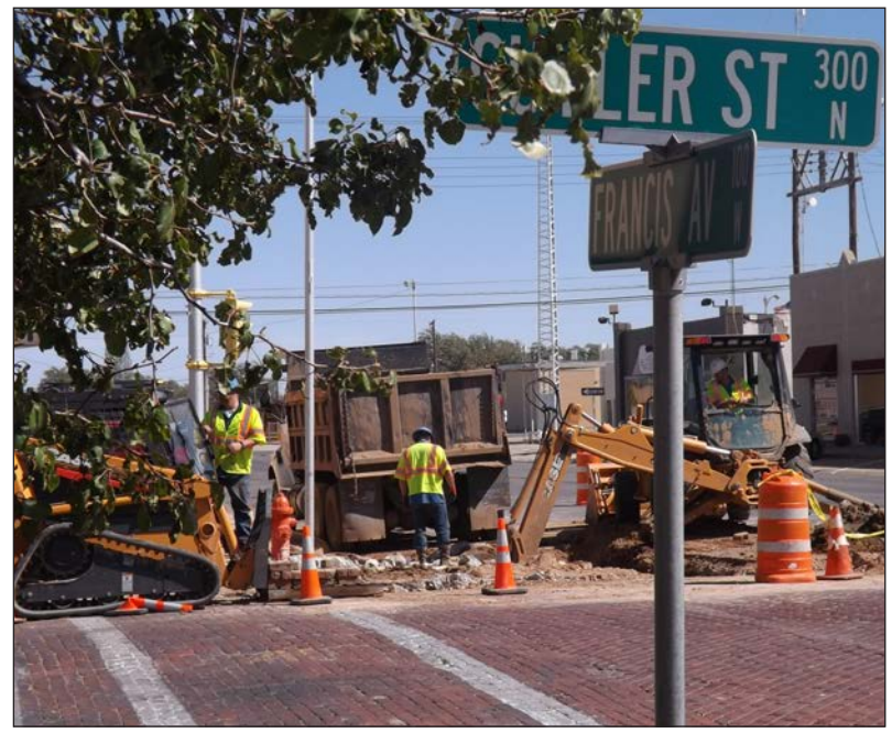
Photo by John Lee City employees work on the northeast end of the intersection of Francis Ave. and Cuyler St. Construction may take anywhere from two to three weeks to complete this phase of the project.
