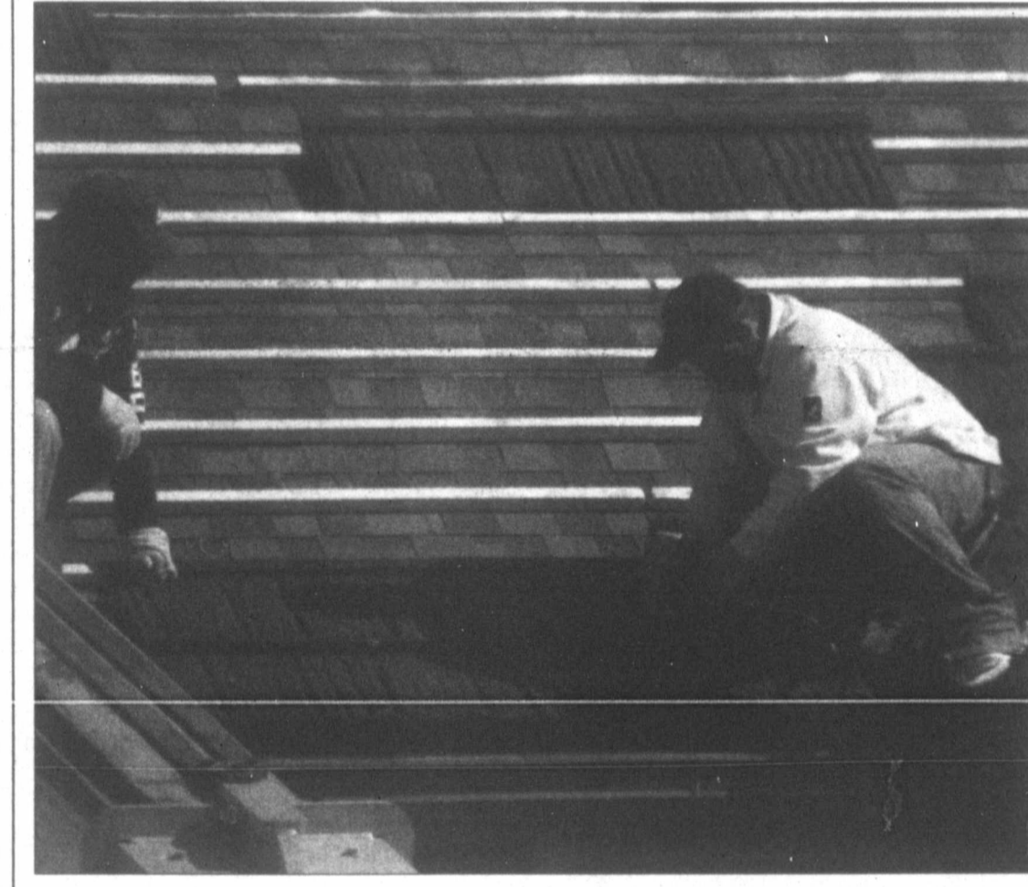
staff photo by Andrew Glover Ivan Ojeda (left) and Julio Leyva of Crawford Roofing lay down stone-coated steel shingles on Mary Ellen and Harvester Church of Christ's roof recently.
