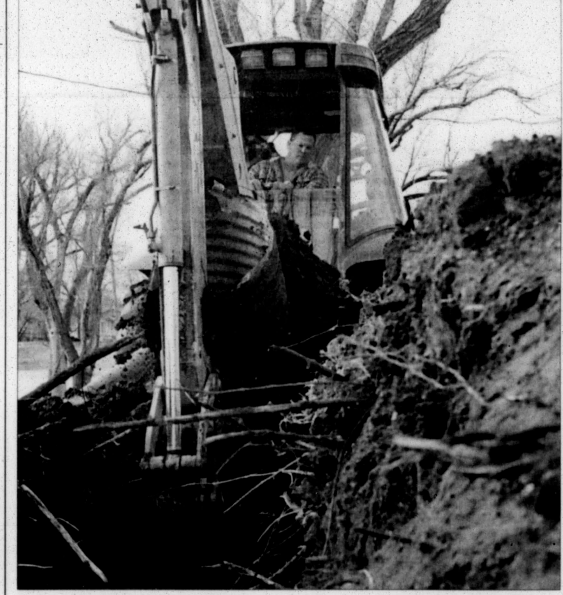
staff photo by David Bowser Jay Weeden pulls an old culvert out of the ground in Central Park as the City of Pampa replaces the pipe that helps drain the park.
