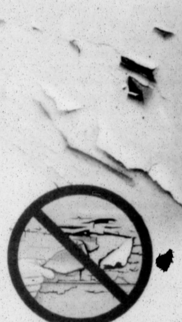
Scraping or sanding lead paint generates large amounts of lead dust.
