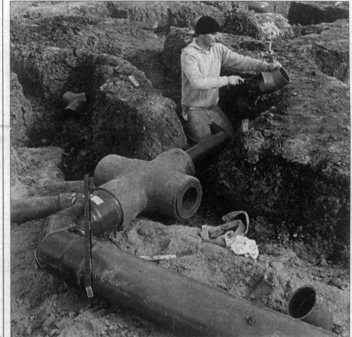
Brad Scott of The Pool Company weaves pipes beneath what will be one of the pools at the water park. Last week's snow delayed some of the work, but crews were still on site this week, as the park is still projected to be constructed on schedule.
