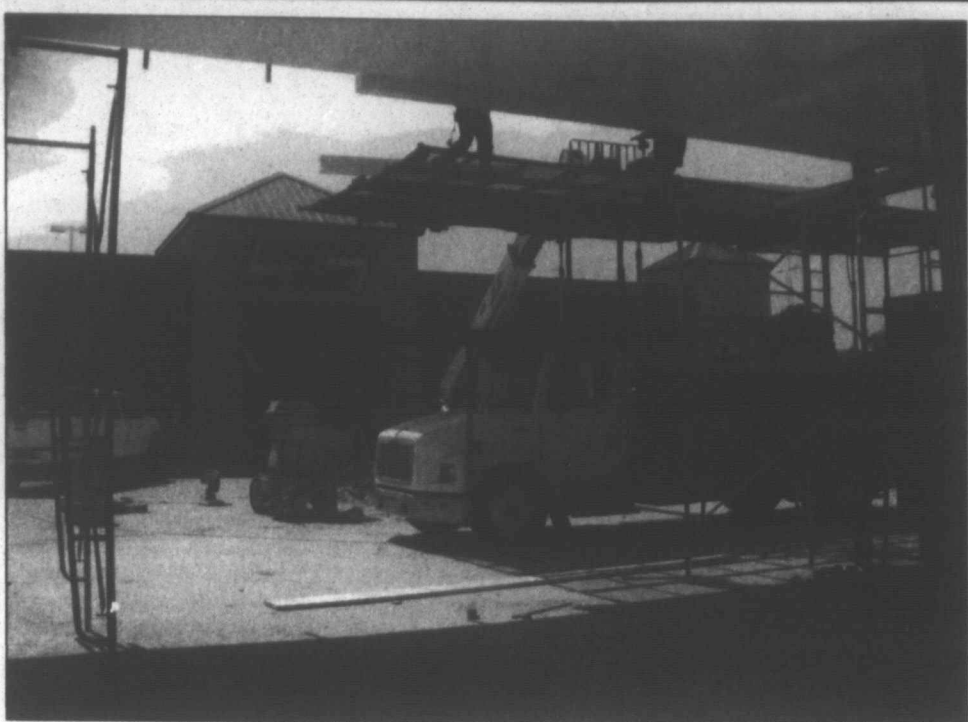
Crews were busy Tuesday finishing work on the canopy and gas pumps at the new Pak-A-Sak store in Pampa. staff photo by Randy Pribble
