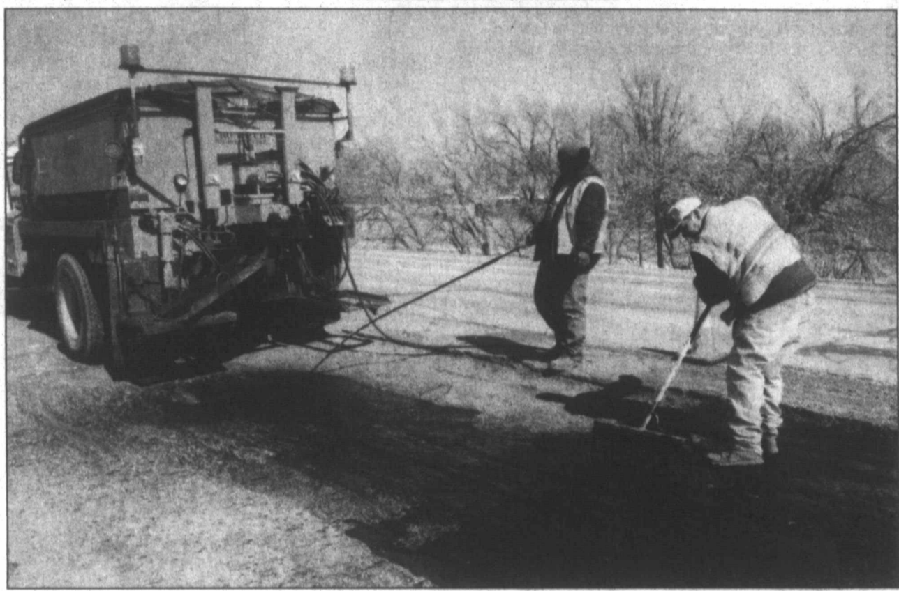
Darron Ellis, left, and James Carson with Pampa's street department worked under blue skies this week after more than two months of harsh winter storms rolling through the panhandle to repair utility cuts in the pavement of city streets.
