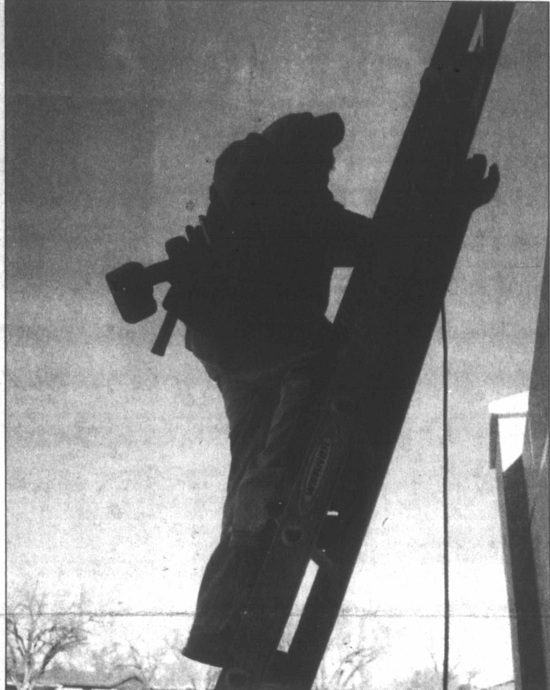
Joshua Castillo with Vasek Services Heating and Airconditioning is silhouetted against a bright blue Monday morning sky as he climbs a ladder to his office atop the new convenience store at Hobart and 18th.
