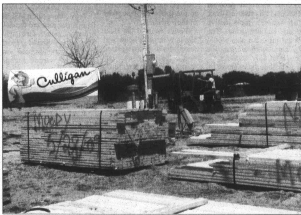
Stacks of boards arrived last week, as volunteers began work on a home for the Carr family of Wheeler, who lost everything in the fire on April 2. The home is scheduled to be completed by Saturday, June 6. Photo courtesy Culligan Water Conditioning of Pampa
