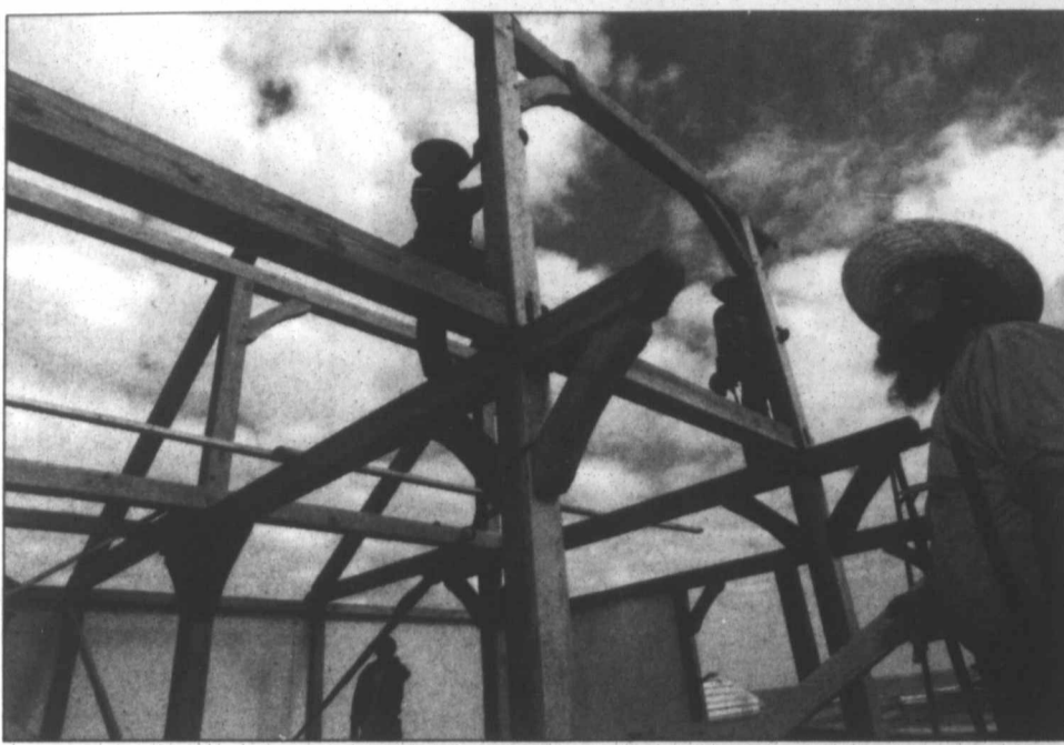
Brothers Pete Schwarz, center top, and Emanuel, second right, maneuver beams as their father, Danny Schwartz, right, an Amish builder from Missouri, directs from the ground in Crystal Beach, Texas on Wednesday, March 4, 2009. Schwartz is visiting Crystal Beach to help rebuild the two story beach home of Blake Rising using traditional Amish style framing. (AP Photo/The Beaumont Enterprise, Dave Ryan)
