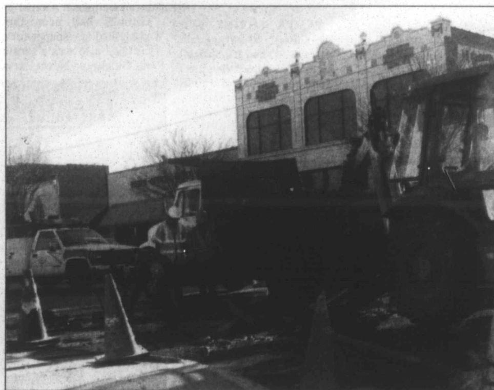
Crews worked to replace a broken water line Friday afternoon at the intersection of Cuyler and Francis streets. The break caused minor flooding on surrounding streets. The crews had to remove the brick paving of the streets and dig to access the pipe, then replace the brick stone by stone after completion.
