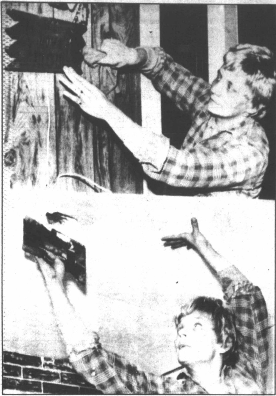
Penny Capstick is shown repairing the damage to her dreamhouse caused by unusual December floods at Times Beach, Mo. The resident of the dioxin-tainted town says the isolation and depression her family feels in the wake of the double disaster has affected them psychologically. (AP Laserphoto)
